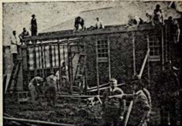
A Working Bee Erecting a hall to house the rapidly growing kindergarten section of the Bible school at Edwardstown West, S.A.
