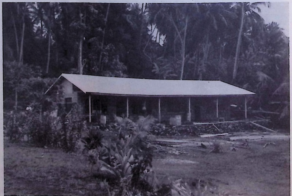
In September a party of workers from the Nunawading, Vic, church, helped to build living quarters for teachers at the Londua Training Centre on Ambae Island in Vanuatu. Here the building is shown nearing completion
